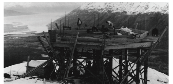
The Roundhouse at Alyeska Museum Archive The original construction of the Roundhouse.
